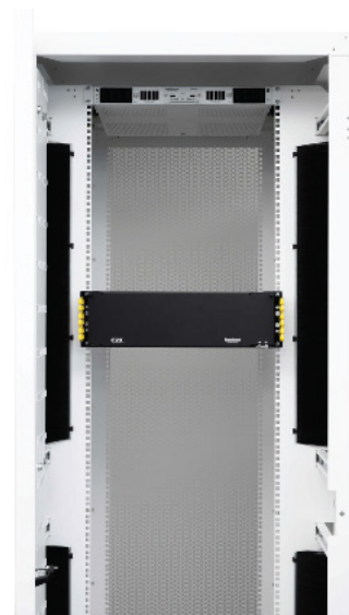
Front view of Data Center Rack with Power Panel and Fiber Panel
