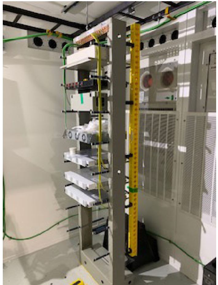
Interior View - Racks
