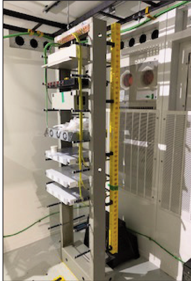
Interior View - Ericsson Racks
