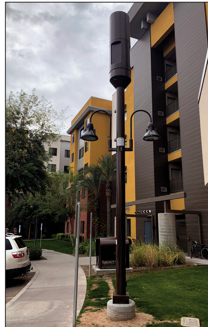
SHRD5 Deployments are Inconspicuous and Aesthetically Pleasing in Municipal Settings
