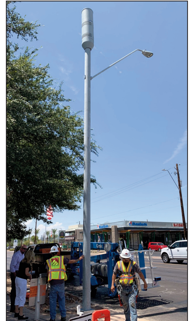
SHRD1 FIELD INSTALLATION
