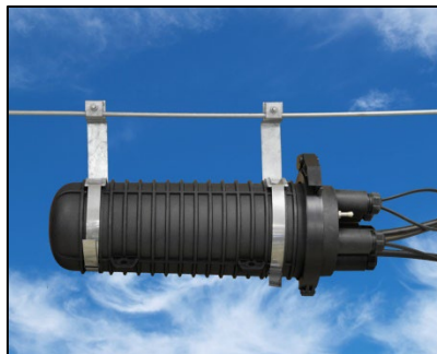
Figure 8 Aerial Mounted FODCB
