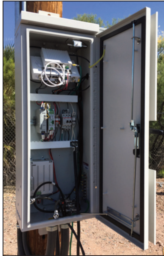
CUBE-MP4016 Field Installation
