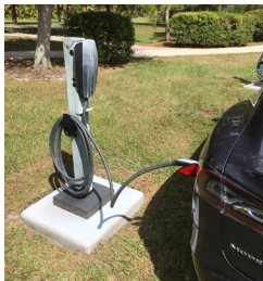
Electric Vehicle Charging Stations
