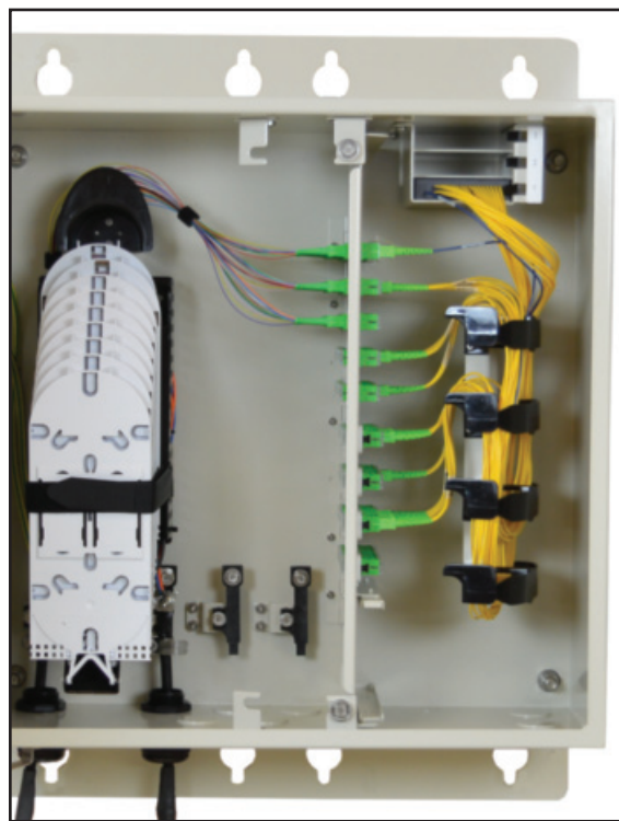
Charles Fiber Splitter Module (CFSM-FM) in a Charles Fiber Building Terminal (CFBT).
